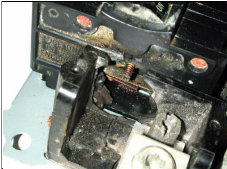
FIGURE 9 - VIEW DOWN TOWARD UPPER RIGHT OF PANEL SHOWN IN FIG. 8. THE FPE STAB-LOK® TWO-POLE 30-AMP BREAKER FED THE CLOTHES DRYER.
