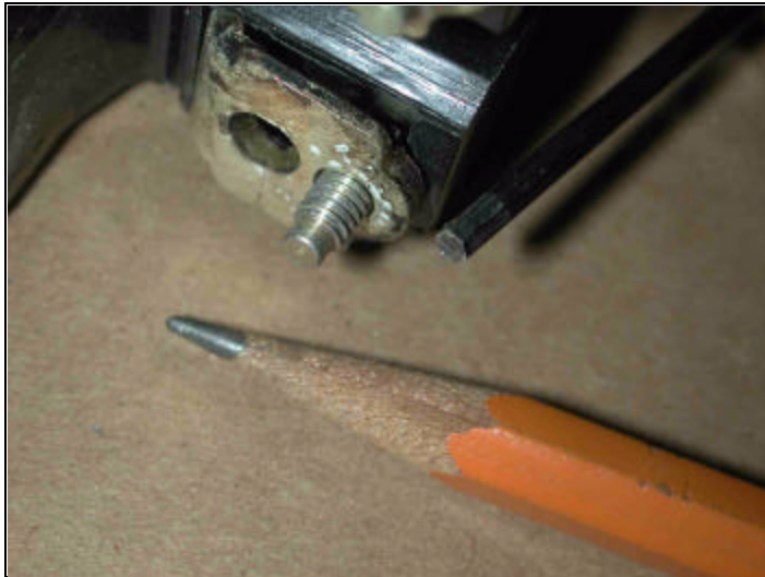
FIGURE 7 - ONE LOAD-SIDE CONTACT AND ITS 8-32 CLAMPING SCREW, ON THE FPE 100-AMP MAIN BREAKER OF FIG. 6. THE SCREW-HEAD TAKES A 3/32" ALLEN WRENCH, WHICH IS ONLY SLIGHTLY LARGER THAN THE LEAD OF THE #2 PENCIL.
