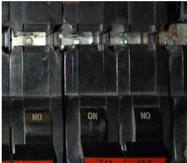
FIGURE 5 - THE ENDS OF THE SCREWS HOLDING THE STAB SOCKET PLATES ARE VISIBLE BETWEEN THE TWO ROWS OF BREAKERS. THIS IDENTIFIES IT AS A PANEL OF THE TYPE SHOWN IN FIGURE 2-C
